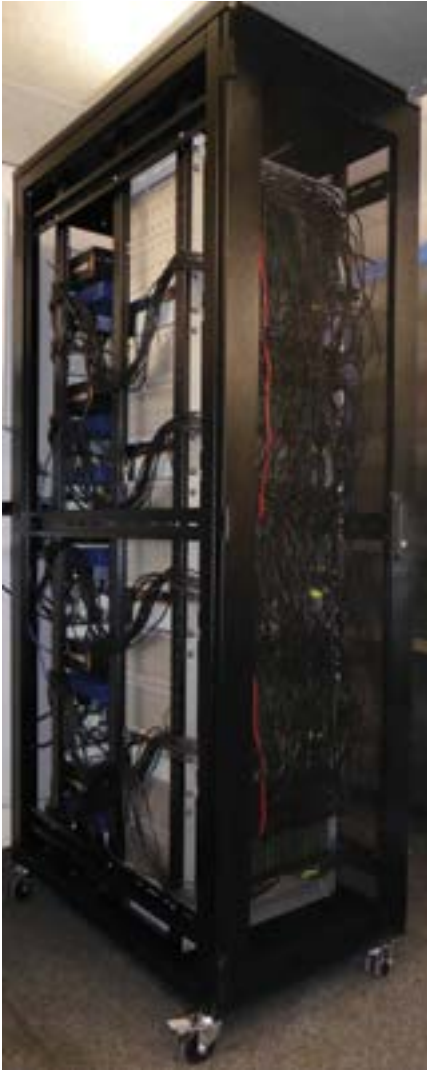
Figure 3: A 19-inch rack incorporating 120 SpiNNaker boards, totalling over 100,000 ARM processors.
